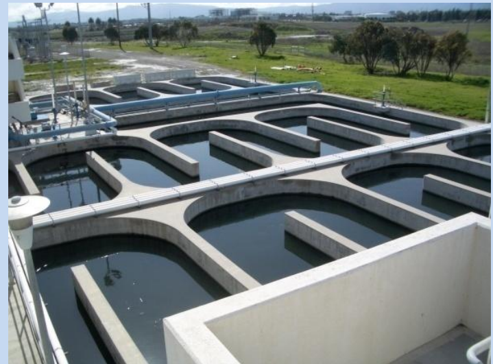
Photo: J. Franco – City of S. Jose WWTP
