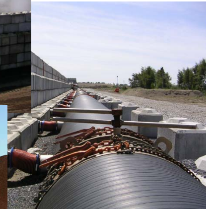
Ventilation to biofilter
